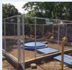
3. Biodigestor reactor biogás
